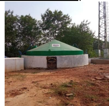
Main Digester Tank (50 Cu M)
